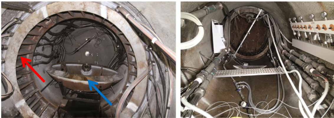
Figure 4. To the left a picture from installation of the plug, the collar is installed (red arrow) while the cap (blue arrow) is on the floor prepared to be lifted and welded in position. To the right a picture from the outside of the test section with the plug in position and all cabling connected.
