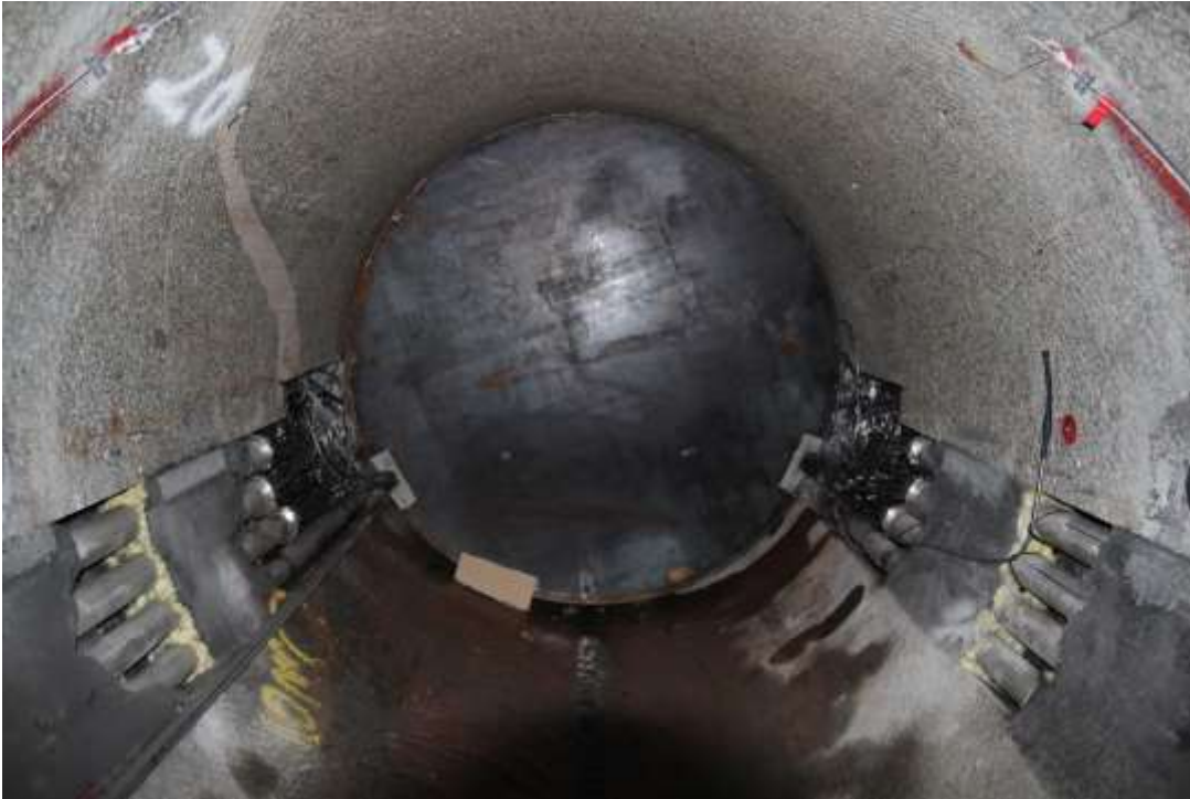
Figure 1.11 Supercontainer positioned in the drift with all its cables pulled. The tight fit between the Supercontainer and drift wall is clearly visible.
